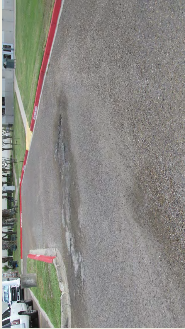
Looking South to North - Pavement damage due to parking lot flooding
