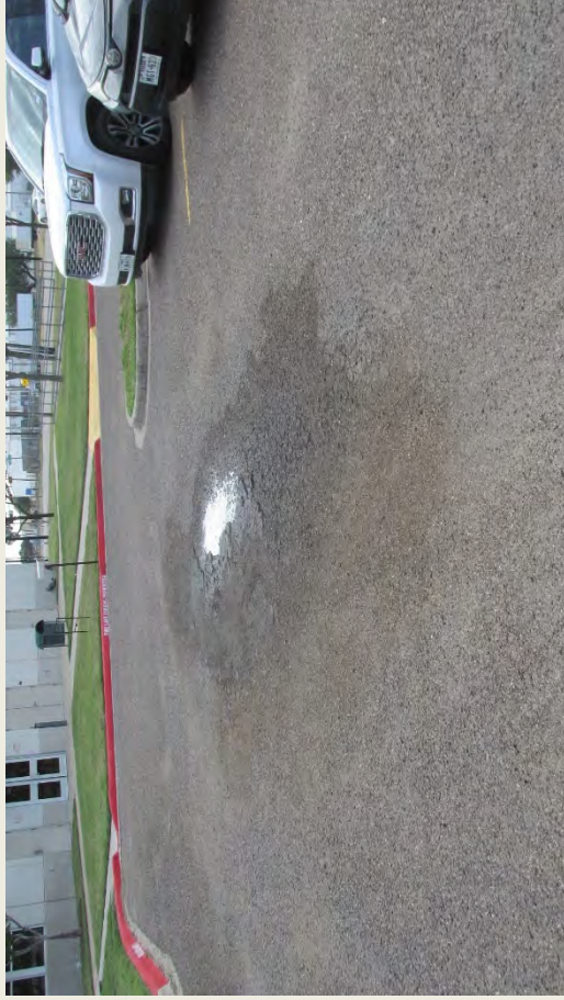
Looking East to West - Pavement damage due to parking lot flooding
