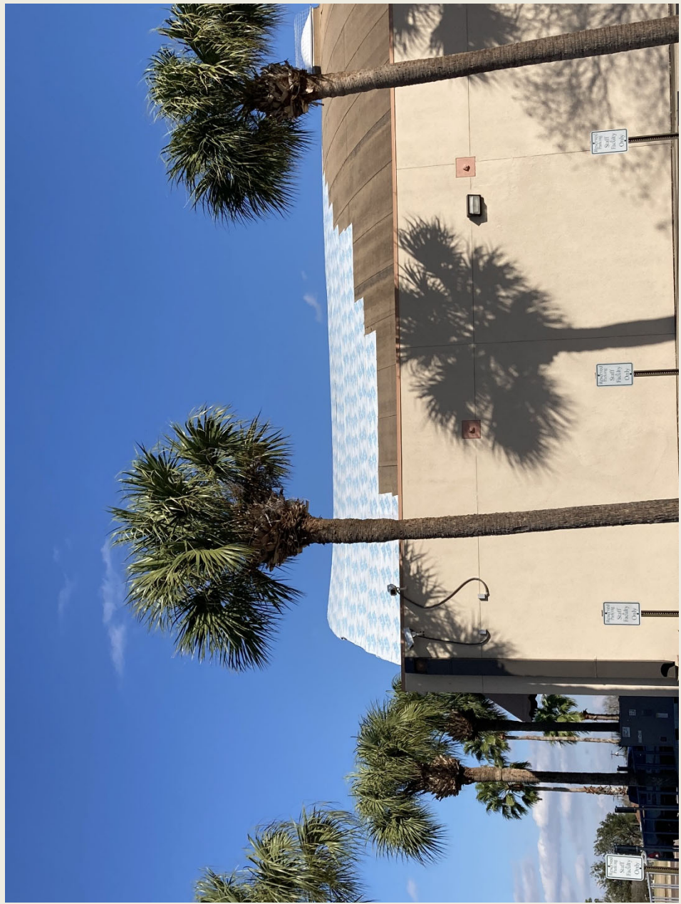
Roof Damage as of 01/31/22
