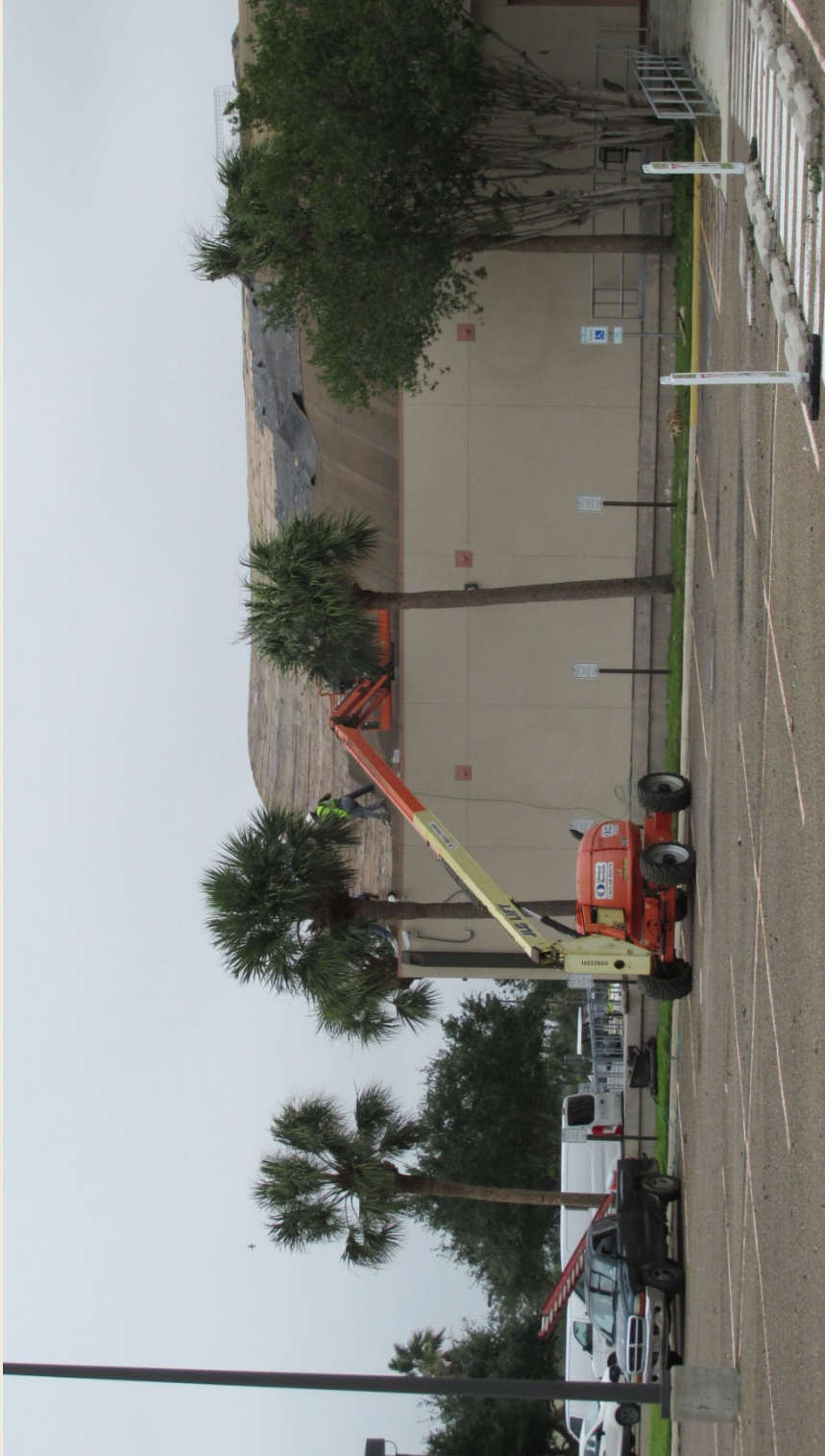
Original Roof Damage
