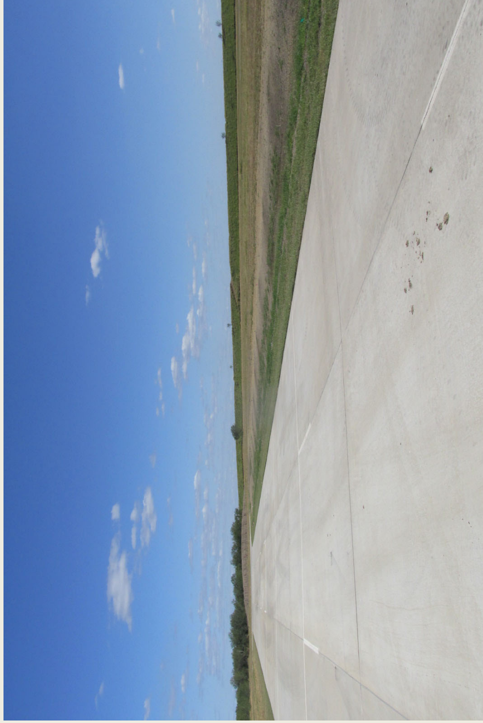
Installation of Skills Pad and Emergency Vehicle Operator Course (EVOC) Site Lighting
